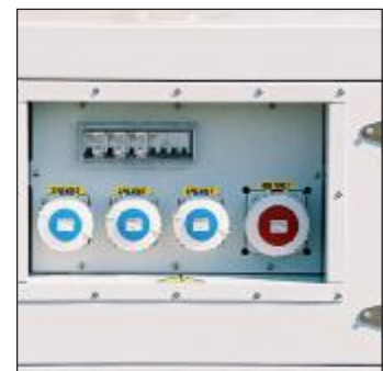
MCBs plus socket outlets
