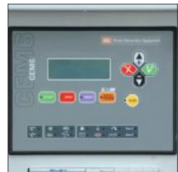
Generator control panel
