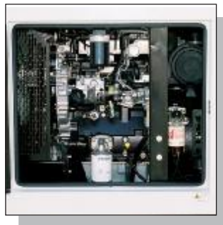
Easy access for maintenance
